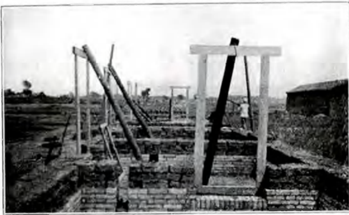
Fig. 90.—Foundation of dwelling, consisting of hard-burned brick; balance of wall to be sun-dried earth brick, seen in Fig. 89.
