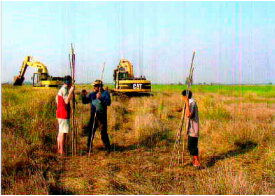
The edges of the letters are marked with poles, so that work with the excavator can begin.
