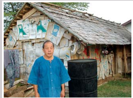
Figure 26. Corrugated paper from old boxes is used for the walls and ceiling. These carton box materials are already over 3 years
