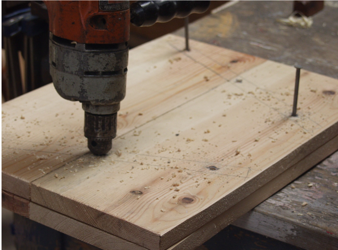
Nails dropped into screw holes maintain positioning while drilling clearance and bolt holes.
