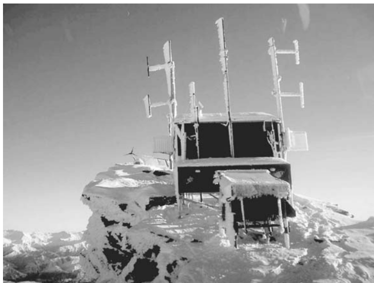
Figure 10.1b Example of a remote VHF facility (Remarkables, New Zealand, this site has helicopter access only).
